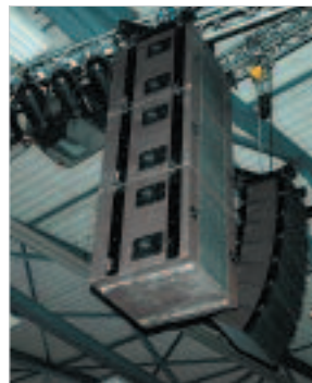
Line Array dV-DOSC von L-Acoustics.
